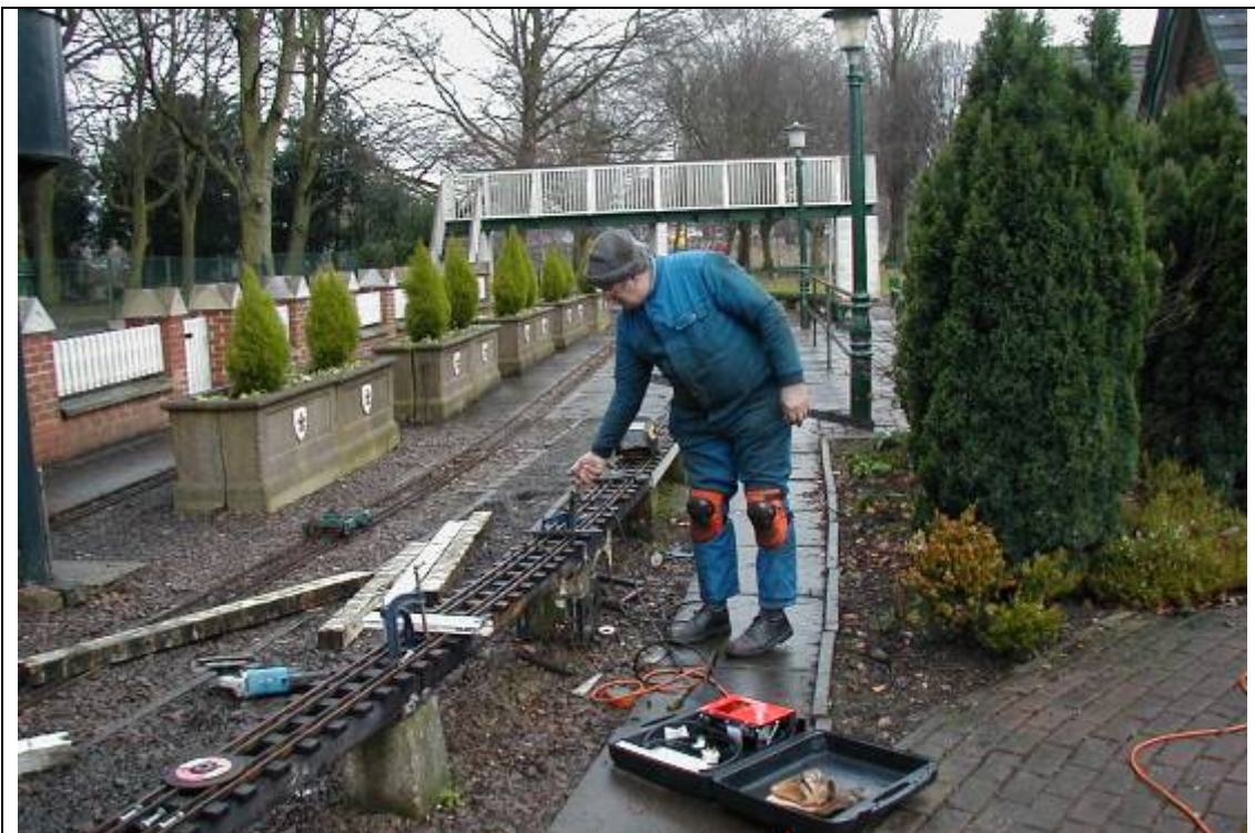
Steve works on replacing the last of the timber on the top track. Work on the raised track should be complete for the 2010 running season
