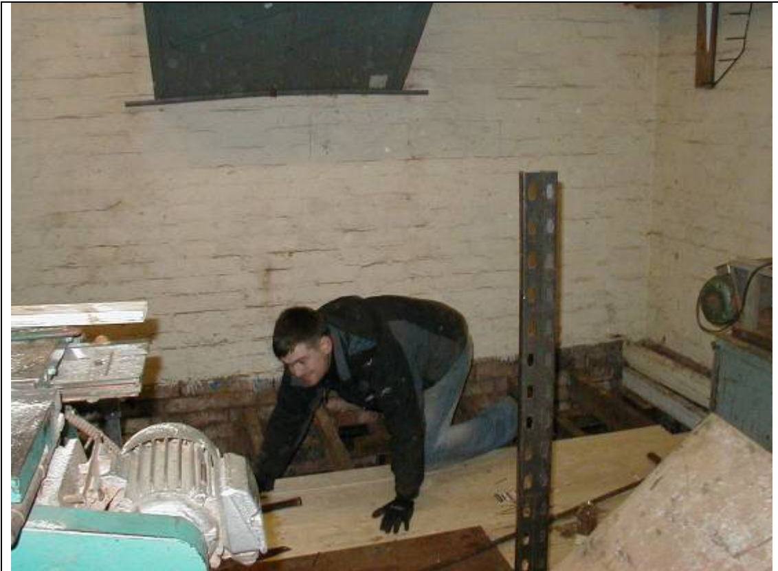
Throughout the winter the rotten floor in the Pavilion building has been replaced. Rob laying floor boards.
