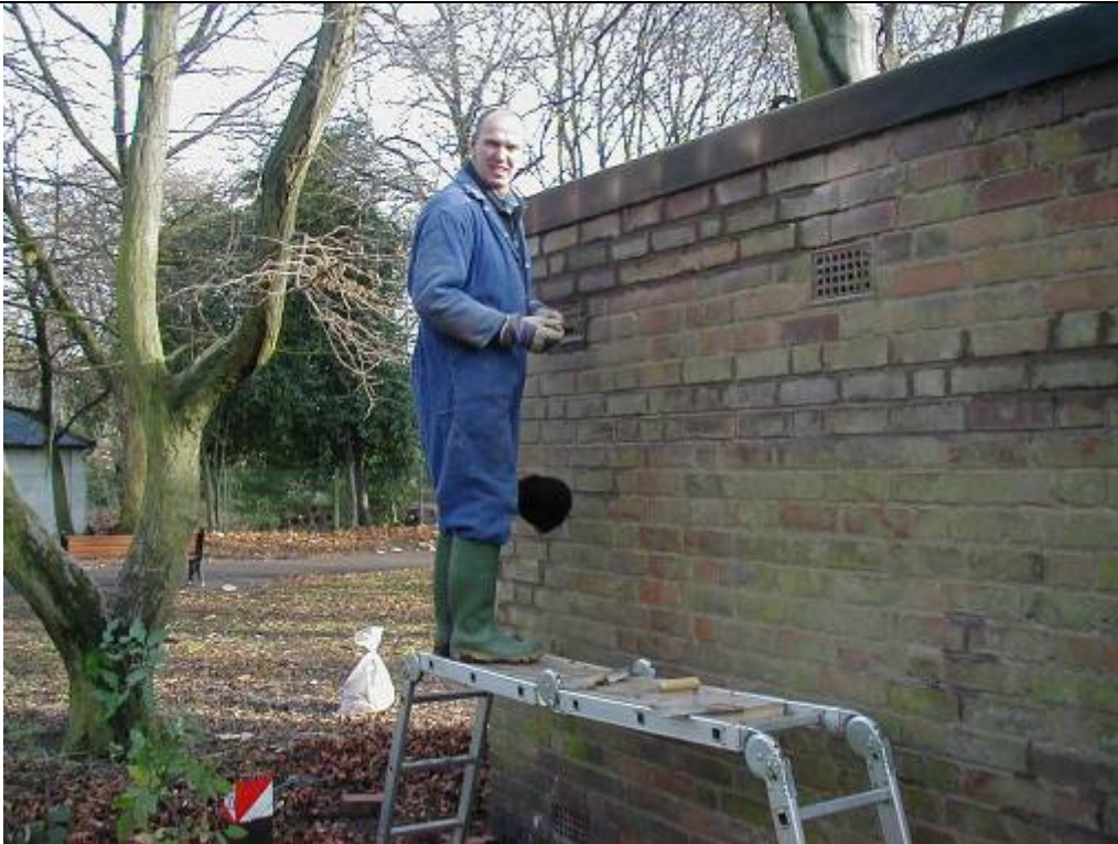
John re-points the brickwork on the mortuary building after it was struck by a falling tree
