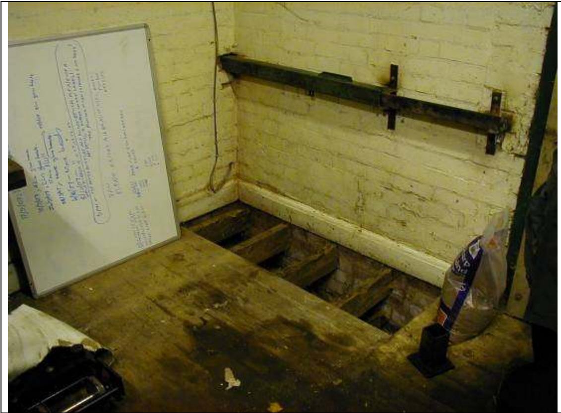
The work bench in the workshop has been relocated as the floor beneath is rotten.
